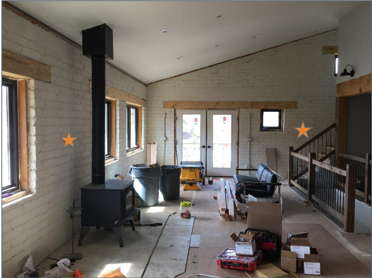
Image 13: View of the Great Room while the building was about to be completed. The two stars show the approximate location of the sensors embedded in the South wall (left), and in the West wall (right).
