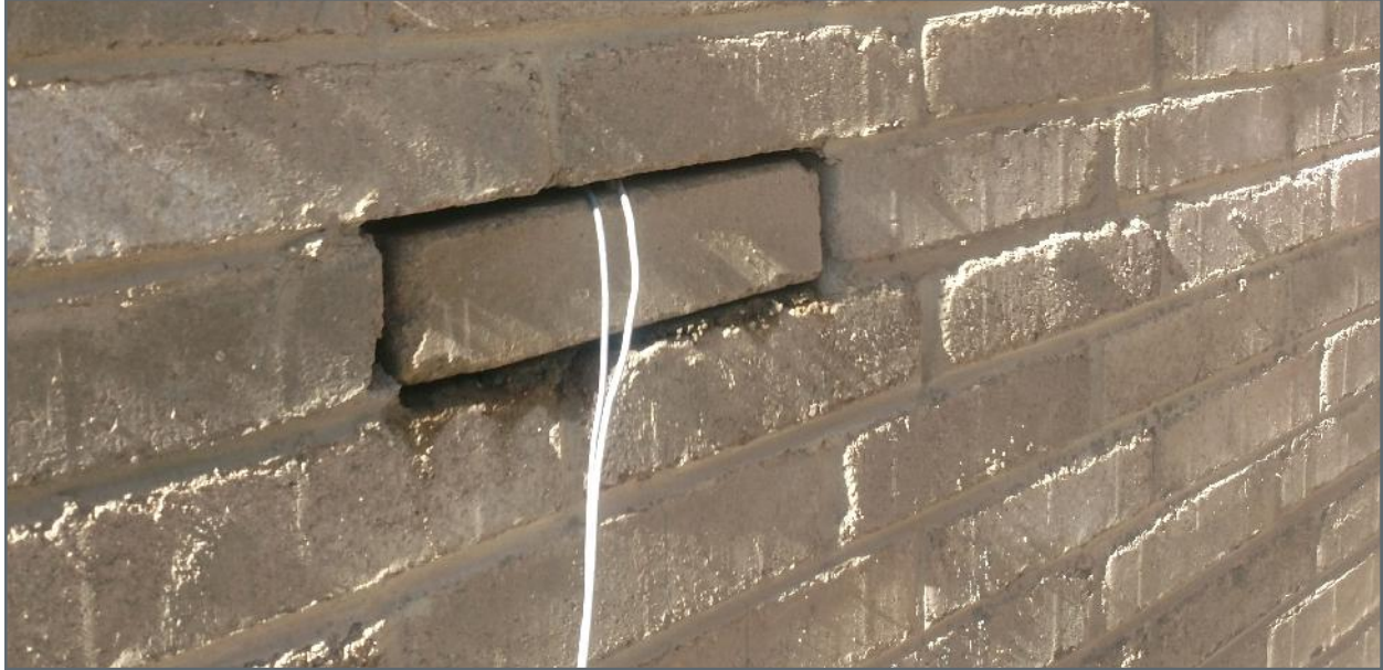
Image16: A CEB block equipped with the embedded sensors, as installed in a CEB wall in the Castle Rock project.
